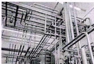
Industrial pipe lines
